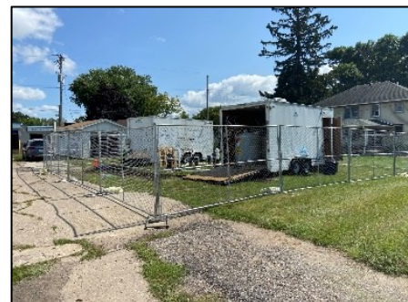
EK-ISCO Pilot Test System at Winona Site
